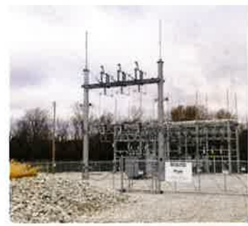
New Carthage Substation
