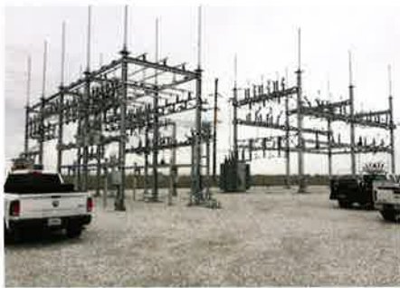
New Elvaston Substation
